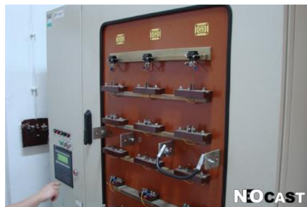
Jumper cable in the course of the investigation. Current load: 750 A
